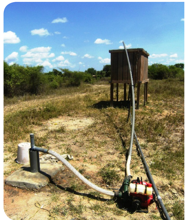
Figure 10 water storage for motor pumpset
