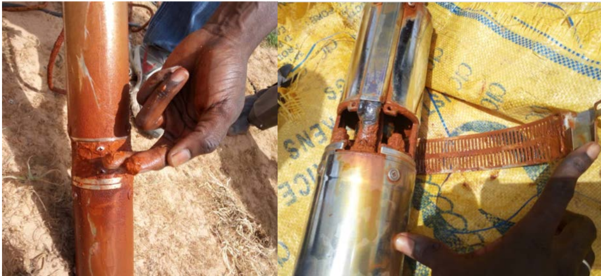
Figure 9 Sludge deposits on elements of the pump
